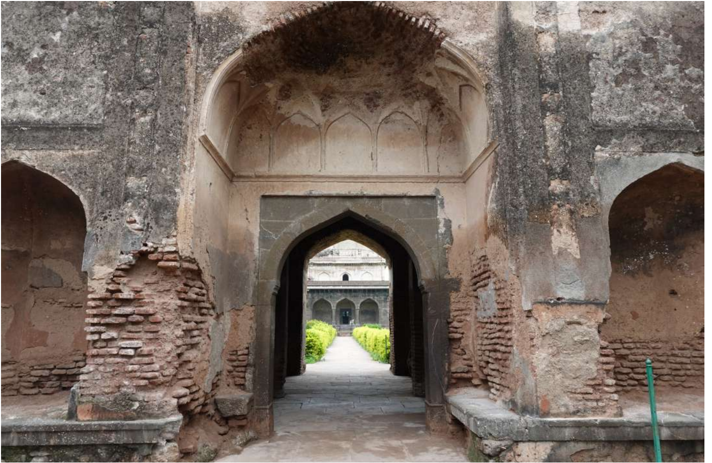
Figure 12 - Entrance gate in dilapidated condition.
