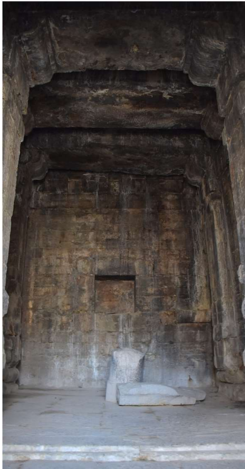
Image 18: Water stains, efflorescence, blackening and tilted beam inside the garbhagriha.
