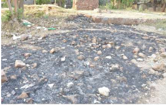
Image 15: Unpleasant view of poorly maintained site close to the Tomb and Gateway.
