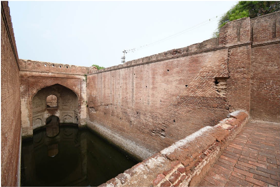
Image 22- Missing of bricks and big cracks on the wall.
