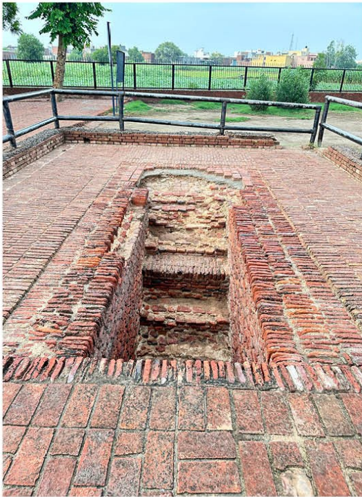
Image 19- Missing of bricks at the entrance of the staircase on northern side.
