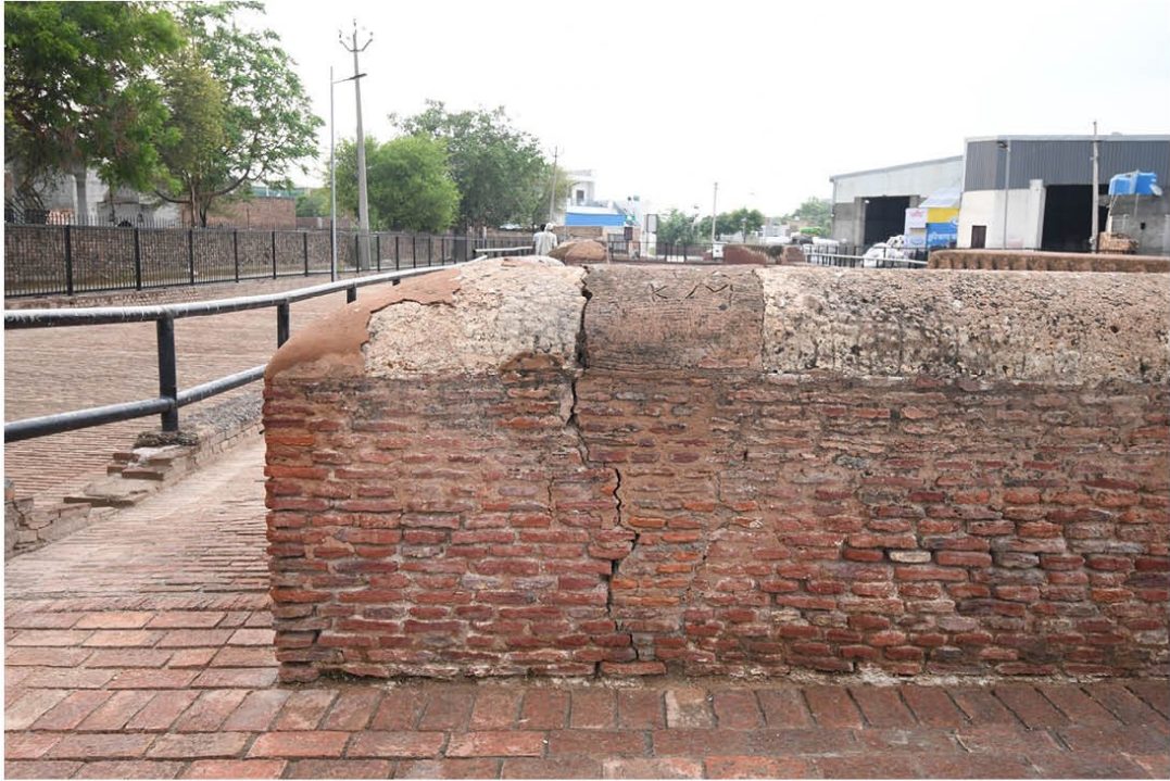
Image 21- Cracks on the parapet wall of baoli
